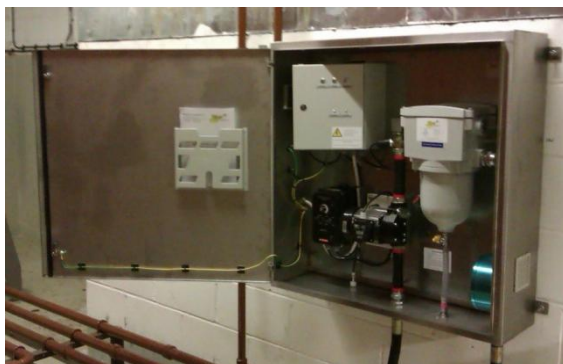
Figure 2: The system installed at the clients facilities
